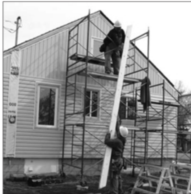
Albert Genaille (roof) and Larry Babcock (ground) put the finishing touches on a newly renovated Yorkton home. Providing adequate and affordable housing in the region was the theme for the Chamber's Regional Housing Conference.
